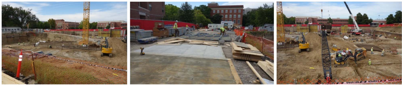
Fig. 3. Images from the construction site that was used as the experimental setting.
